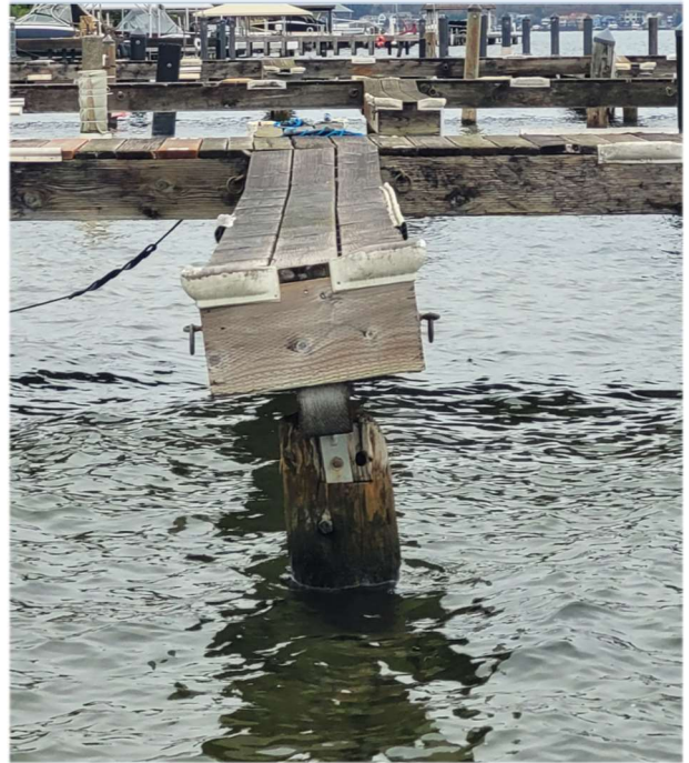
Unstable/leaning finger pier
