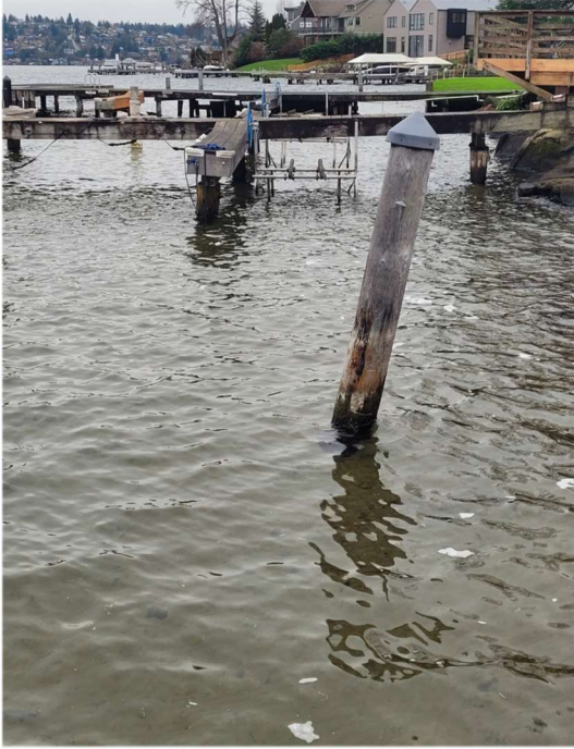
Failed mooring pile
