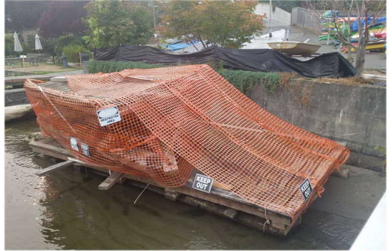
Section of "day dock" retained from 2018 failure
