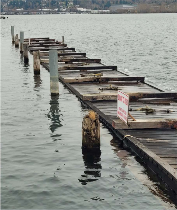
Outer "day dock" in disrepair
