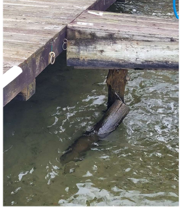
Failed support pile
