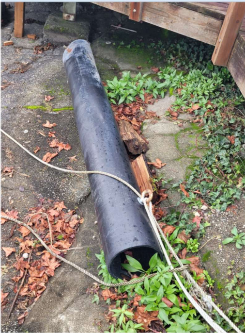
Broken mooring pile, resulting in unusable boat slip
