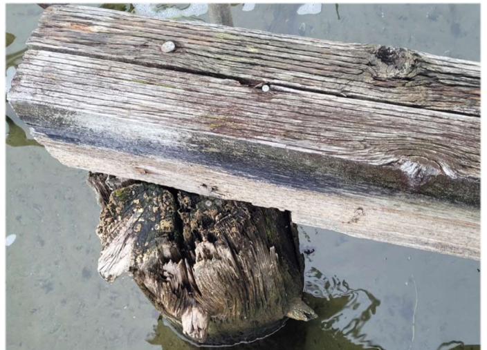
Decaying structural pile
